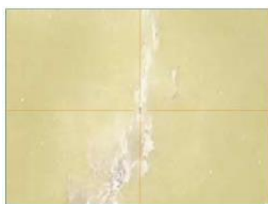
Side view microbe damage.
